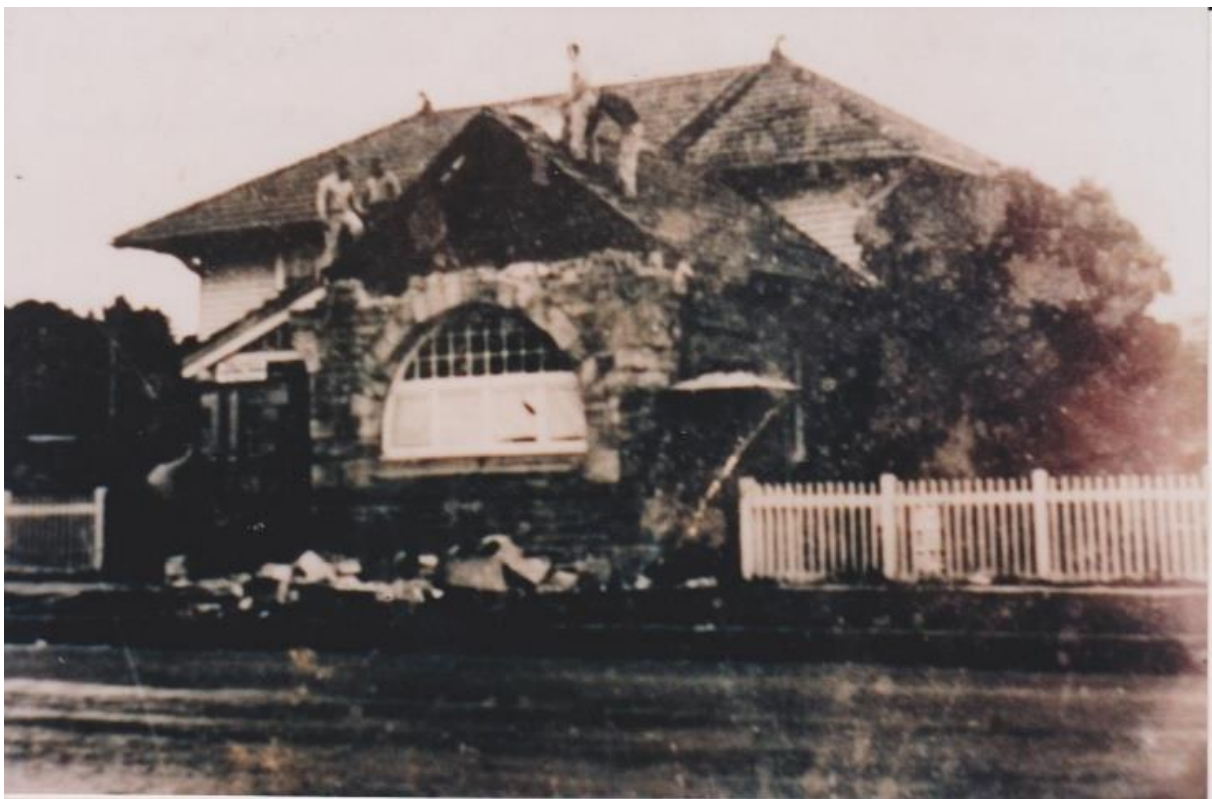
Above: The above image was taken shortly after the Monday 22 May 1961 earthquake showing clearly that the stone chimneys and the stone gable wall above the window have fallen. The front window, the elegant side timber-supported entrance, telephone box and picket fence all still intact (Photo from Debbie Gilroy via the Robertson History Group).
