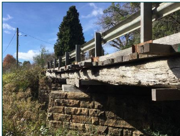
Plate 17: Nattai Creek Bridge showing central pier and existing girders, decking and railing, facing east.
