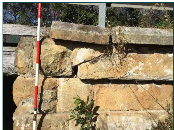
Plate 15: western abutment, facing south, showing vegetation growth, damage to masonry from sinkhole and evidence of repaired mortar work.
