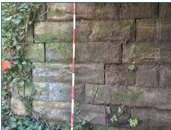
Plate 14: western abutment, facing west, showing vegetation growth and deterioration in stonework.
