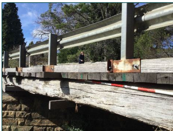
Plate 20: General view of northern side of bridge showing timber girders, replacement deck and guards rails [facing southeast]
